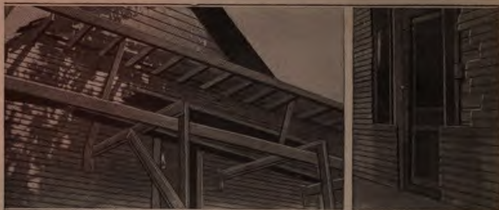
PHOTO COURTESY GROVER HOOVER The Side View Shows the Narrow Weather Boards of the New Structure being Built a Few Inches Away from the Old One. The View of the Front Door Also Indicates the Small Space between the Two Walls, and the Necessity of Having the New Doors Correspond in Position to the Old Ones
